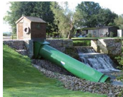
The picture shows an 11kw plant on a river in Somerset from a head of 2.6 metres with a flow of 600 litres a second.
